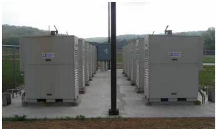
Twenty-four methane-powered Capstone microturbines provide electricity to the Sauk County Landfill in Wisconsin.
