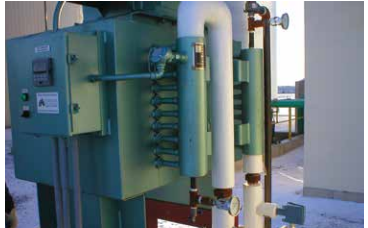
Cain Heat Exchanger for heat recovery from the Capstone microturbine.
