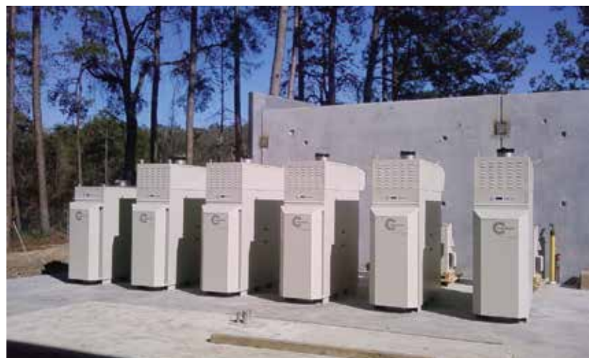
Six Capstone C65 microturbines generate continuous power at this U.S. government office.
