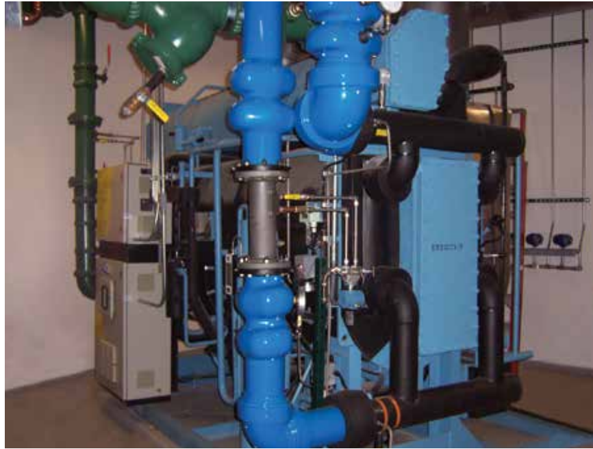
Thermax® absorption chillers.
